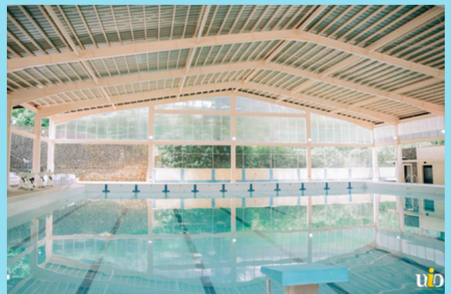
Closed-loop system in Aquatics facility for secondary use of pool water
