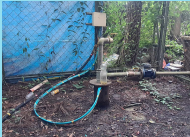
Surface fixtures of the deep-well extraction system in the main campus
