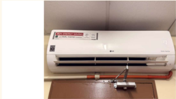
Utilization of air conditioning units with at least 70% of energy saving
